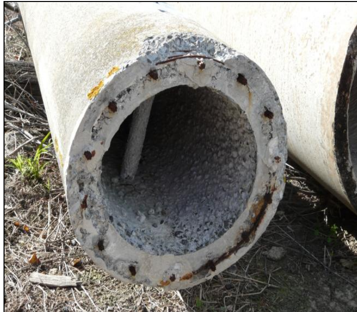
Figure 7: Hollow spun pole top cross-section with cap removed showing ends of vertical prestressing strands, and portions of spiral binding wire
