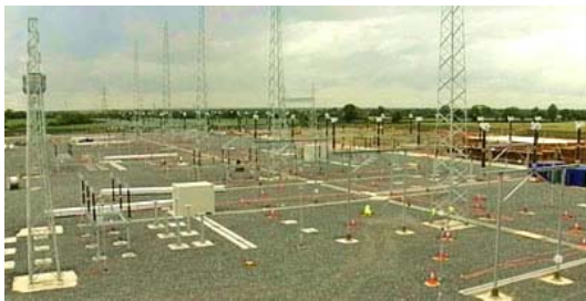
Figure 2: Low profile substation (Source: POWERTEAM Electrical Services)
