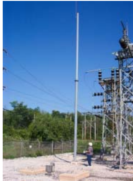
Figure 1: Traditional lightning mast protecting substation from lightning
