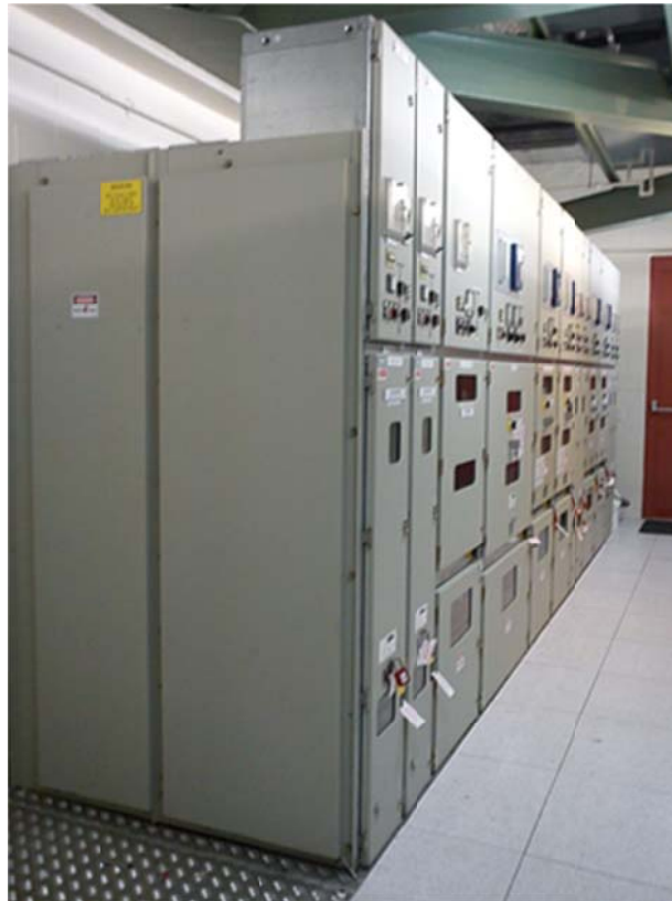
Figure 1: TCC Switchboard Panel
